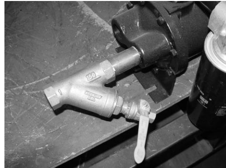
Figure 5 Wye-strainer installed, with cleanout valve.
