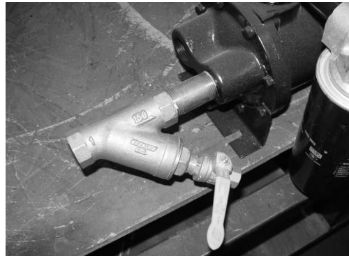
Wye-strainer installed, with cleanout valve.
