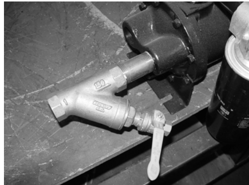
Figure 4 Wye-strainer installed, with cleanout valve.
