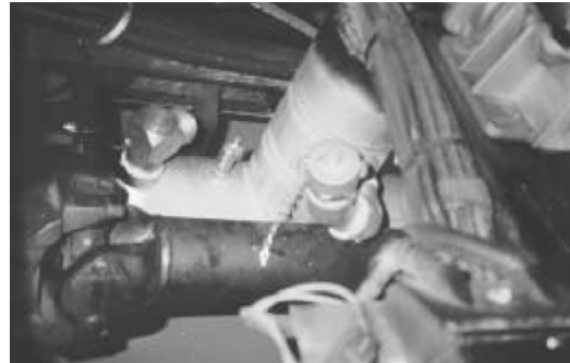
Two elbows on an oil fill cap for accessibility
